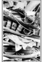
Piles of rubble: Dirty dishes remain stacked near the Garden Room with portions of the ceiling collapsed on them. QZOOM
