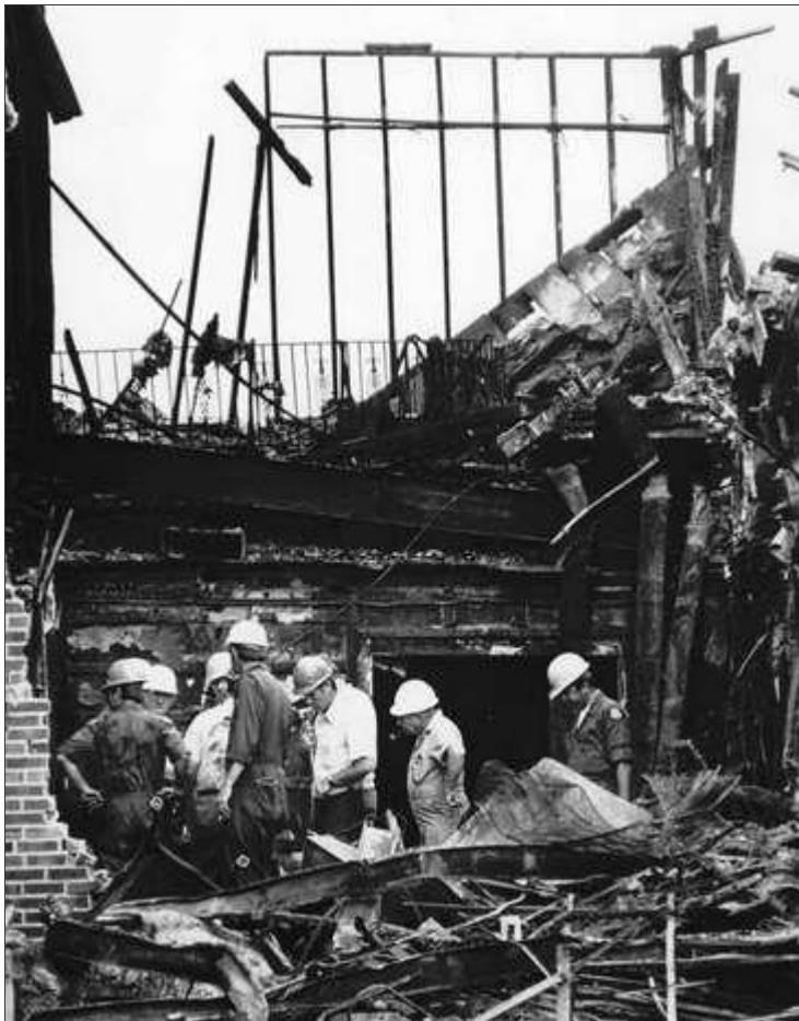
Workers sifting through rubble after the Beverly Hills Supper Club fire - May, 1977.
